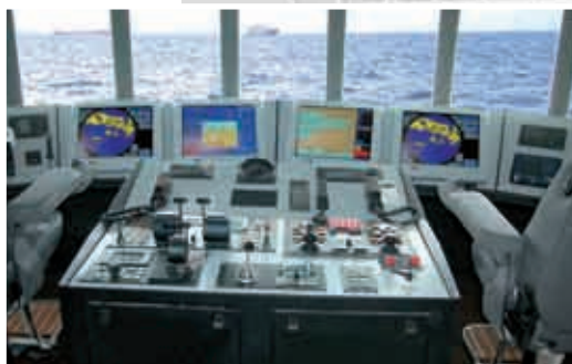
Kelvin Hughes Integrated Bridge System Screen format 4:3
